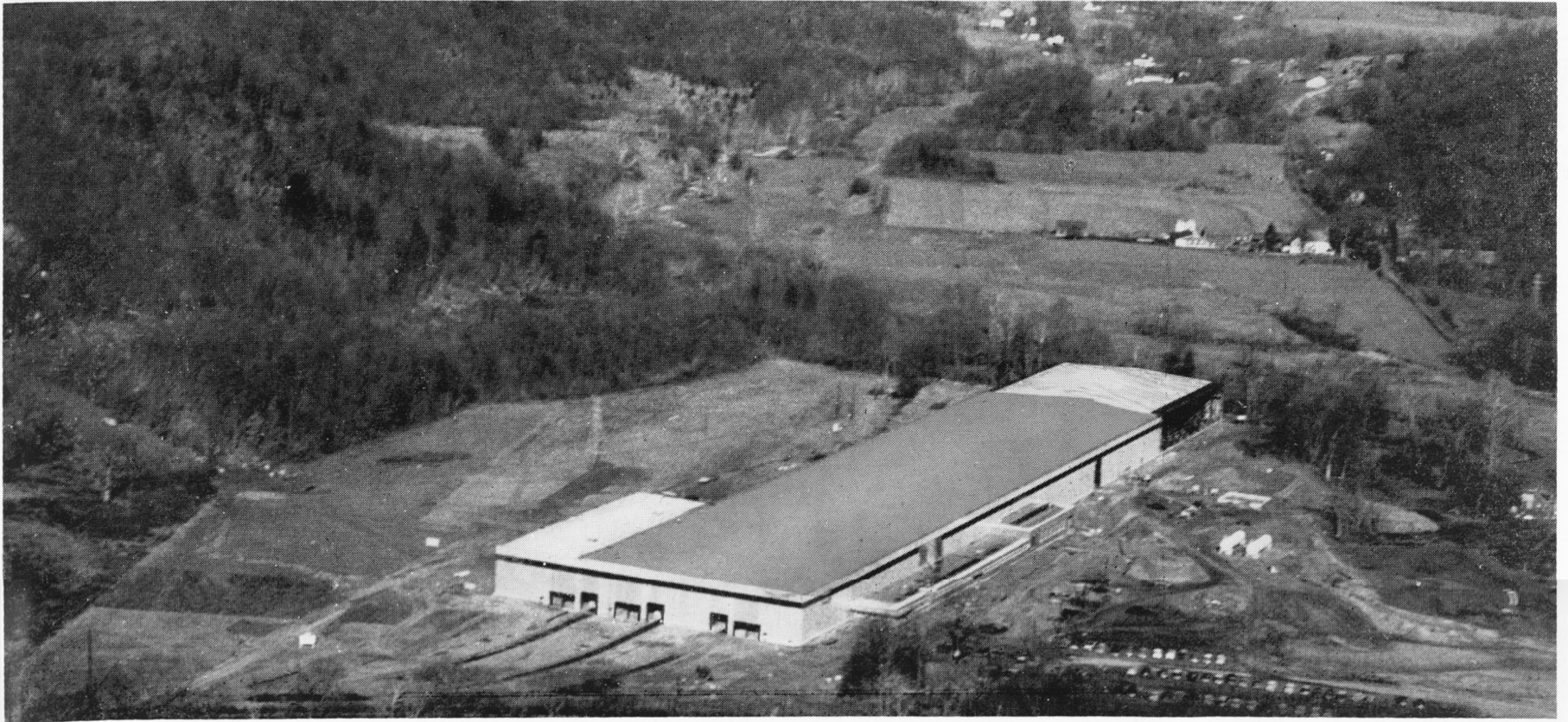
Construction of the Company's new Tube Mills at New Milford is on schedule. The roof and sidewalls are up, ready for the heat to go on.
